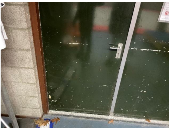
beschadiging binnendeur gymzaal 4
