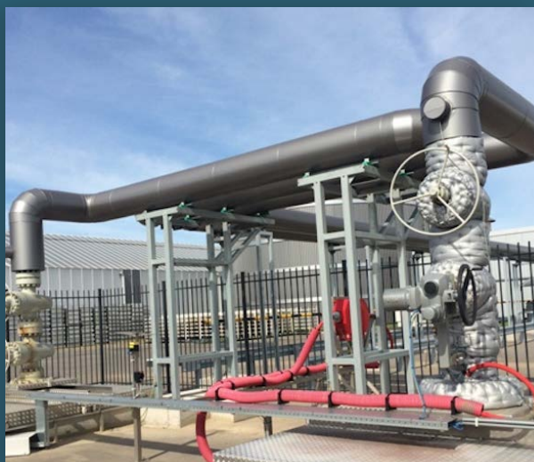
Bovenstation geothermie put 10-30MW
