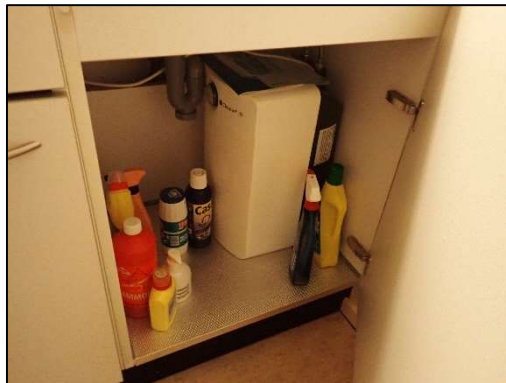
Close-in boiler t.p.v. pantry bibliotheek
