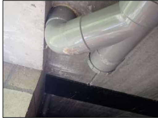
Incidenteel lekkende PVC riolering
