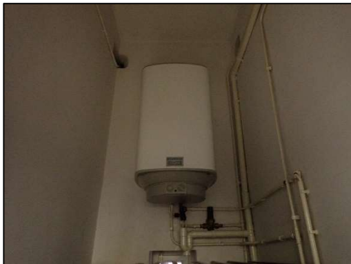
Close-up boiler nabij garderobe
