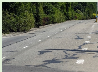
Scheurvorming asfalt (C)
