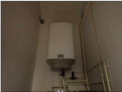
Close-up boiler nabij garderobe
