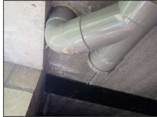
Incidenteel lekkende PVC riolering
