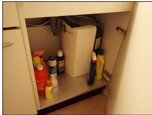
Close-in boiler t.p.v. pantry bibliotheek
