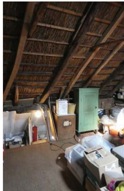
Daksporen boven woning.
