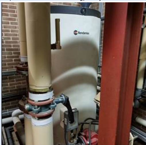
Indirect gestookte boiler 25-meterbad
