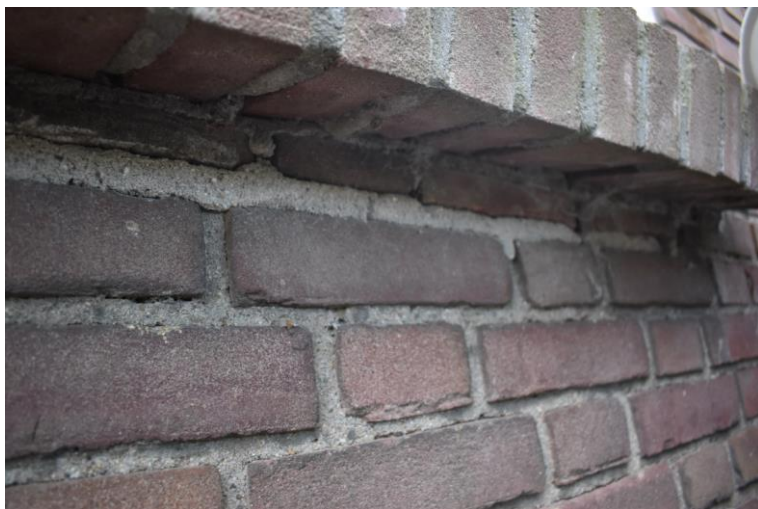
Later ingebrachte bakstenen raamdorpel.
