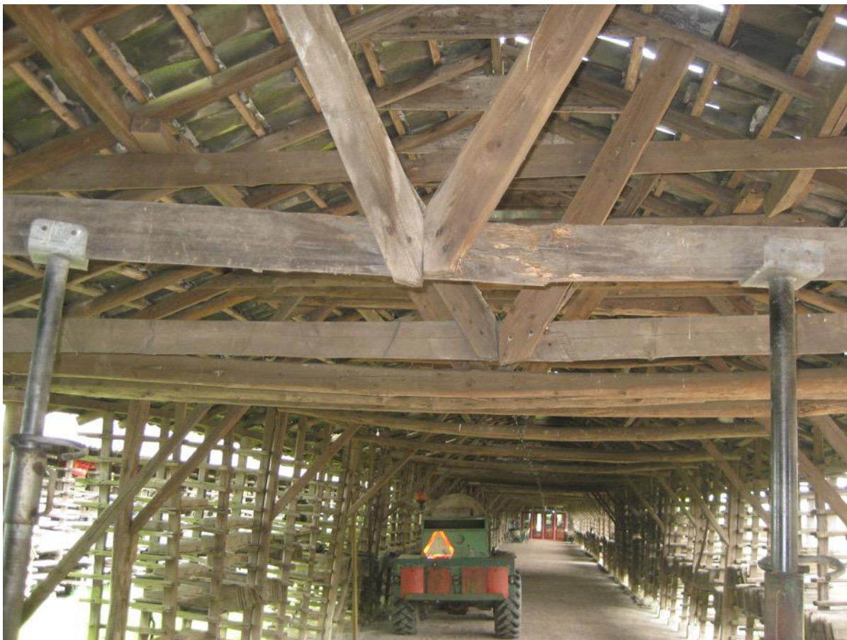
Droogloods 4 gebroken spant
