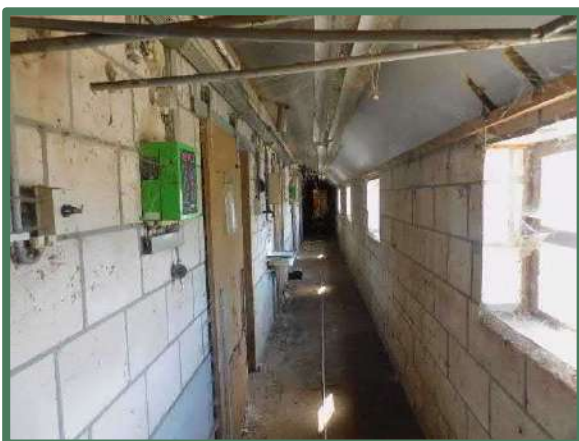
Centrale gang stal 1
