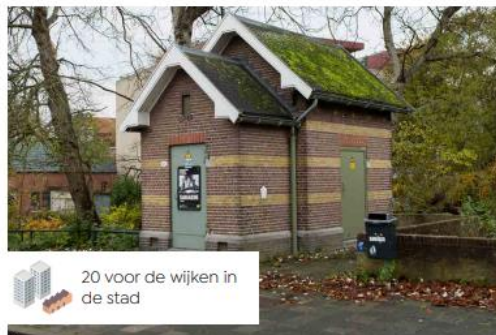
MS-MS station (3-23kV)
