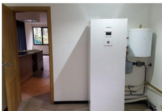
Binnenunit + warmwater boiler
