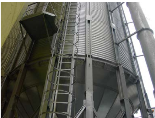
Figure 2: example of a similar, bolted, silo
